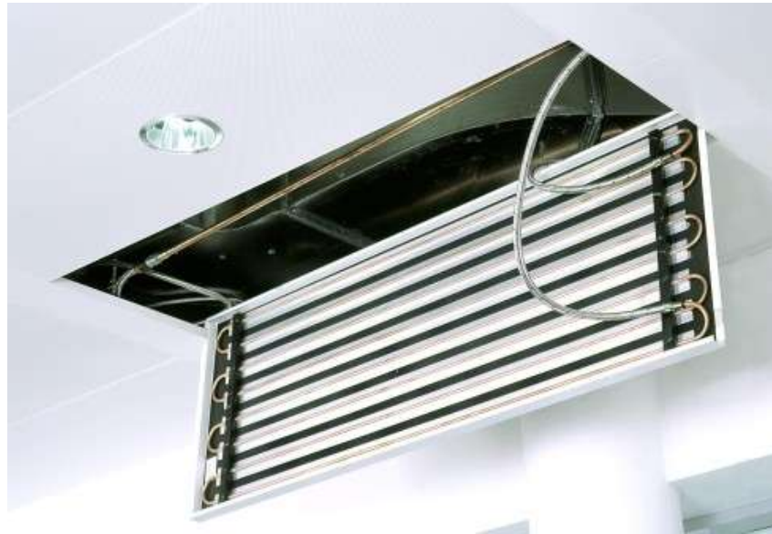
FIGURE 4. Chilled ceiling installation /11/
