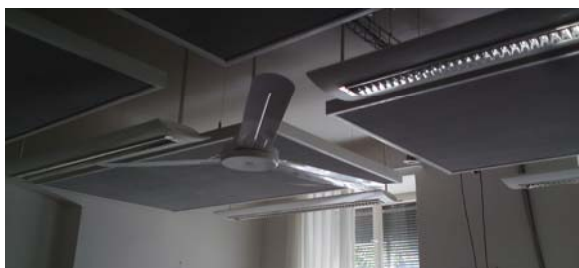
Figure 3: Ceiling fan and suspended ceiling with PCM in R3
