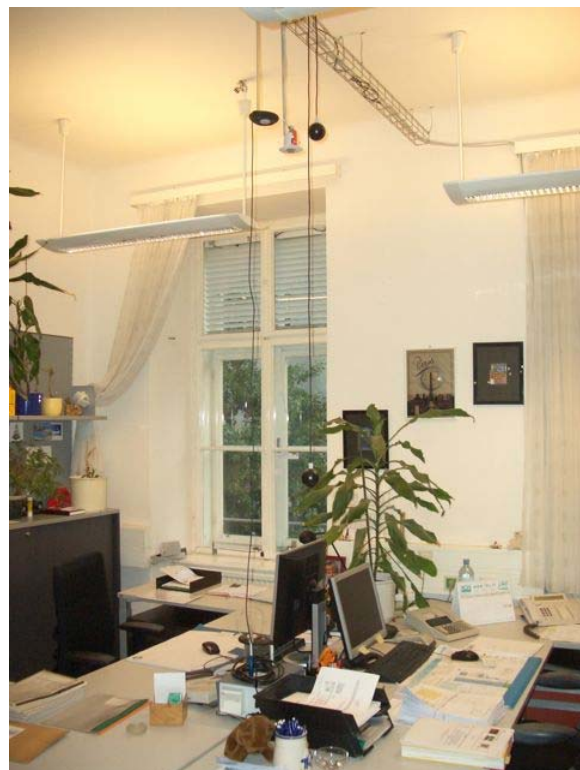
Figure 4: Workplaces in R2 with motorized window, internal venetian blinds and sensors for air, surface, and globe temperature, relative humidity, occupancy, illuminance, wind velocity and carbon dioxide
