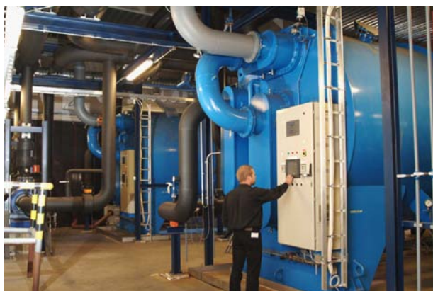
Figure A2.3.3: Installations of Helsinki Energy
